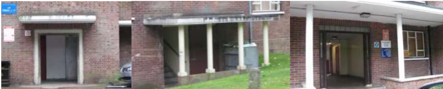
Cumberland House, simple detailing obscured by bin, sign proliferation, unsympathetic light and conduit
