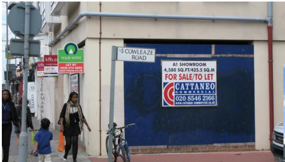
Uncharacteristic, external, wrap-around pipework.....
