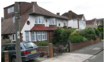
Characteristic roof form undermined
