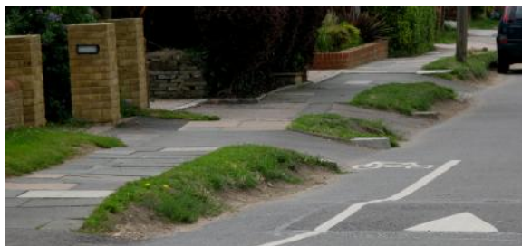
Eroded grass verges and unlevel footpath
