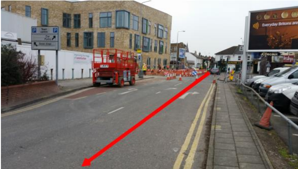
Figure 66 Pipework route along Kingsgate Road towards gas holders site (looking East) at the construction of the new Kingston College building.
