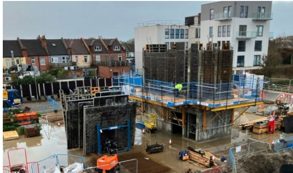
The west core shutters in place ready for the 1st floor pour
