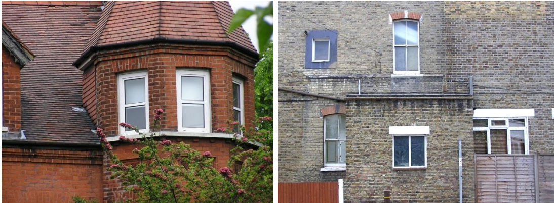
PVCu windows at 29 Kingston Hill and window pick-and-mix at 23 Clifton Road
