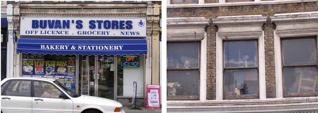
Park Road suffers from inappropriate shop-fronts, and upper floors in poor condition
