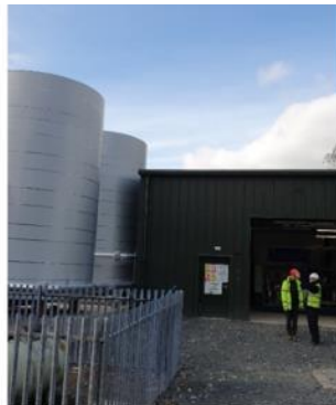
Energy centre and thermal stores
