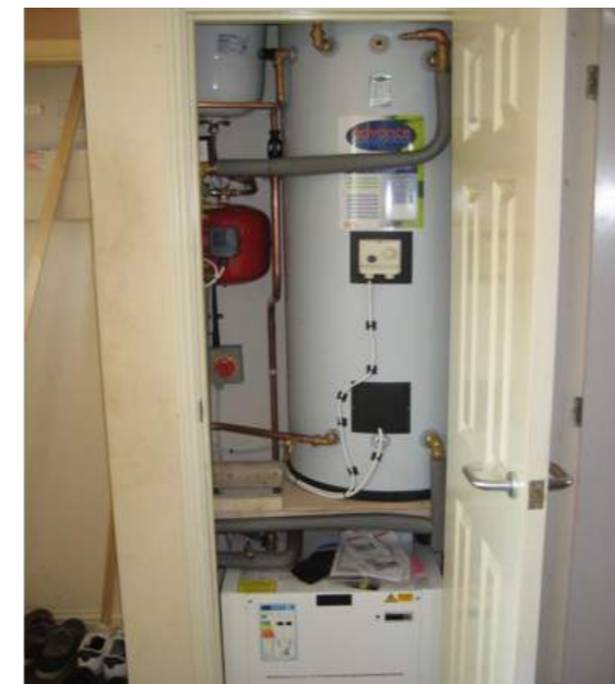
Figure 5.10: Kensa Shoebox individual GSHP installation 26
