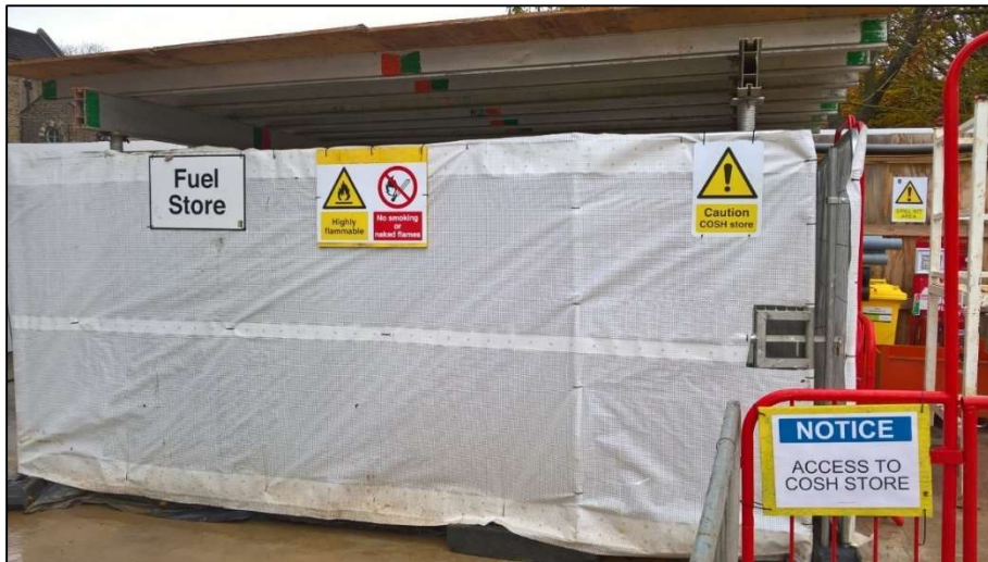
Figure 14 – Adequate signage and control of Fuel Storage
