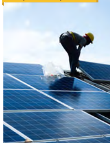
Roof spaces used for photovoltaics
