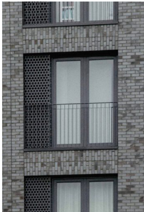
Figure 4.38: Vent panels at Clapham Junction.
