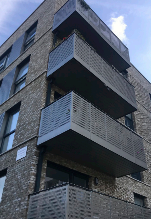
Figure 4.203: Metal balustrading which promotes privacy.
